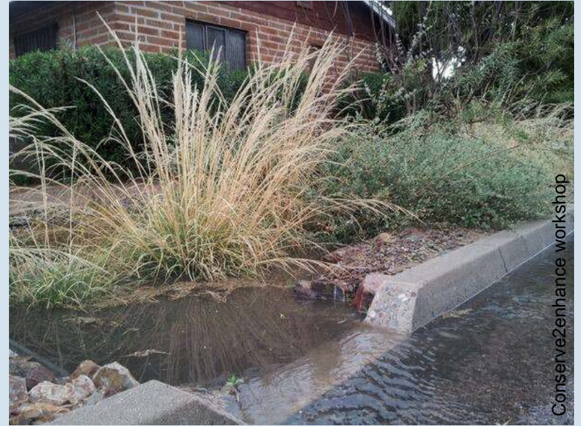
Curb cuts, slope, and swales are combined to direct rainwater to small basins - infiltration areas
